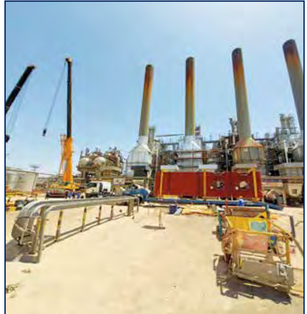
Revamp of Boilers at Mina Al-Ahmadi Refinery for Kuwait National Petroleum Company
