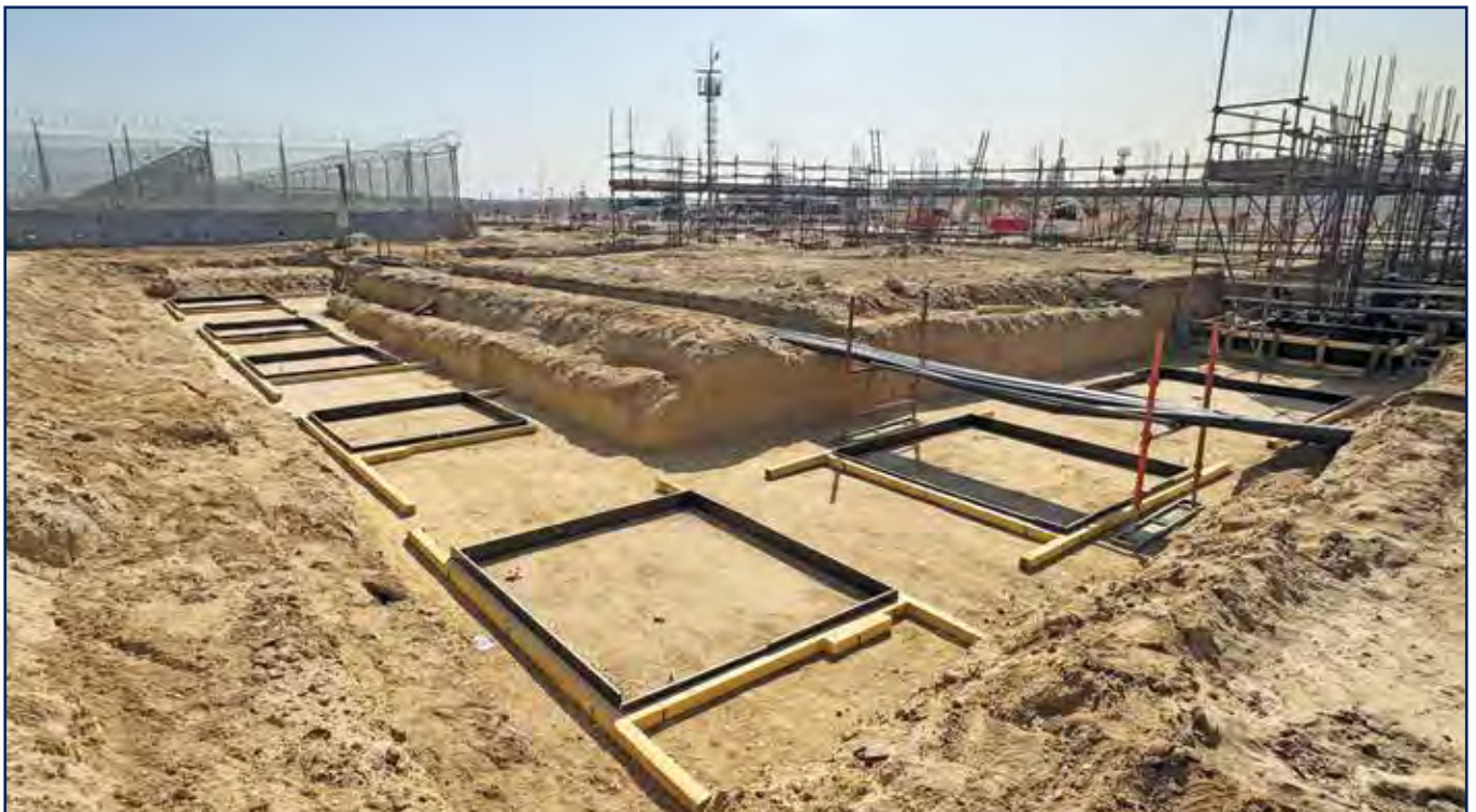
Procurement and Construction for Upgradation / Modernization of Gatehouses at Mina Al-Ahmadi and Mina Abdullah Refineries for Kuwait National Petroleum Company
