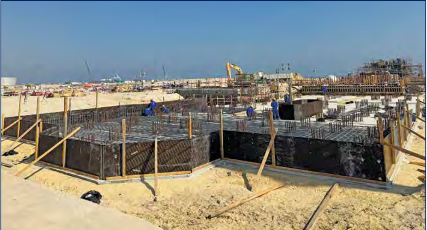
Civil works for the EPC of Qurayya Expansion CCGT IPP Project for SEC, KSA
