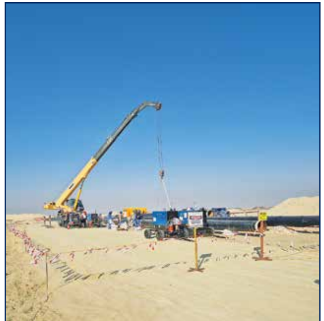
Pipe Welding Works at Gas Condensate Network Project for Kuwait Oil Company
