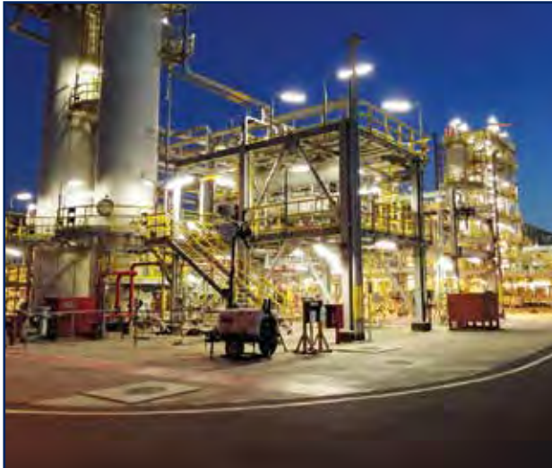
Electrical & Instrumentation Operations
