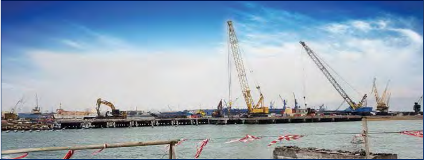
Maintenance and Replacement of Corroded Parts of the Seawater Intake Gates at Al-Sabiya Power Station for Ministry of Electricity & Water and Renewable Energy
