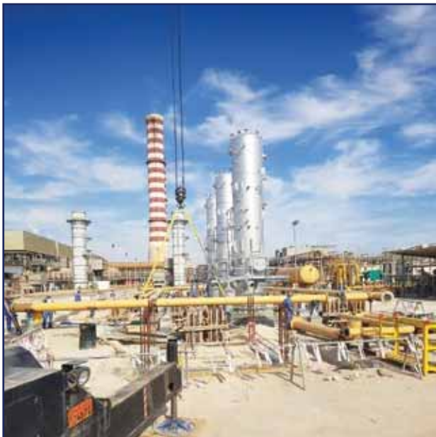
Power Plant Operations
