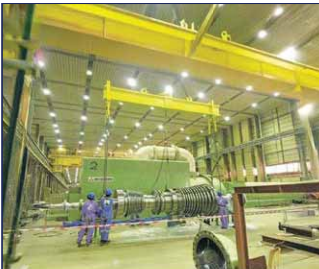
Power Plant Operations
