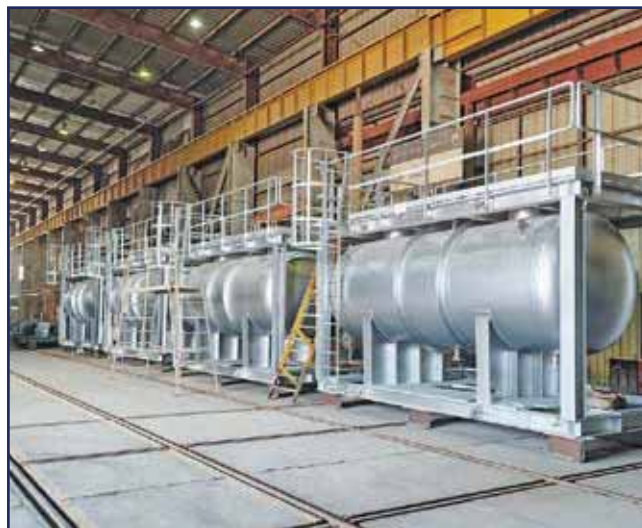
Gas Scrubber Package for Joint Operations - Wafra
